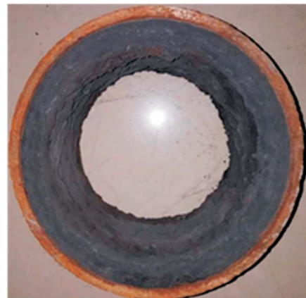
Figure 1. Coal mine drainage pipe scale.
