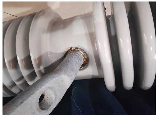
Fig. 11. Failure diagram of cement adhesive in insulator.
